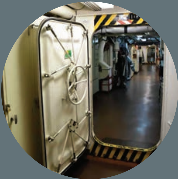
ship watertight doors
